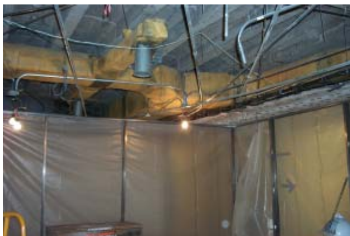
There's not much left of the copy room, with only sheets of plastic where the walls used to be. Photo by Todd Staats.
