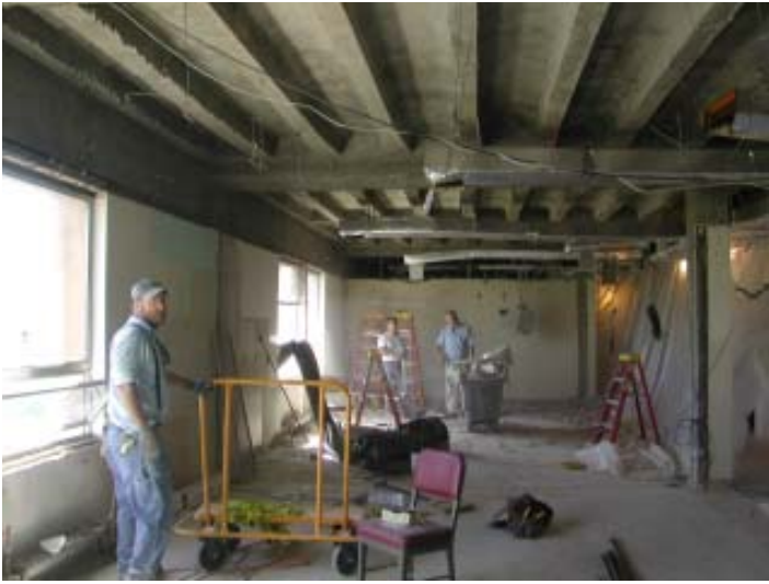
Chris, Rick and Bobby, during the demolition phase of the old music library.
