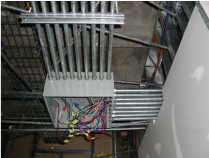
Conduit art: What we found in the ceiling was a rats nest; what we replace it with will be a work of art!
