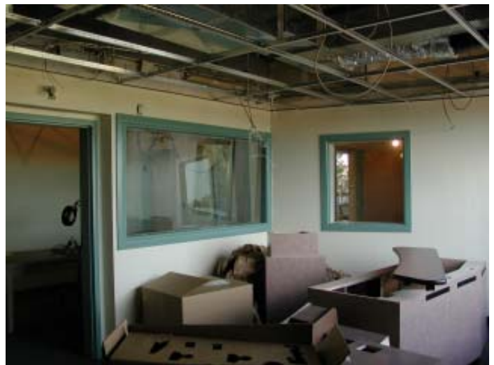
The new control room equipment and console were delivered in October; we’ll spend November on installation.
