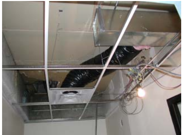
When the ceiling tiles came down, we learned that the heating/cooling ductwork would need to be replaced.
