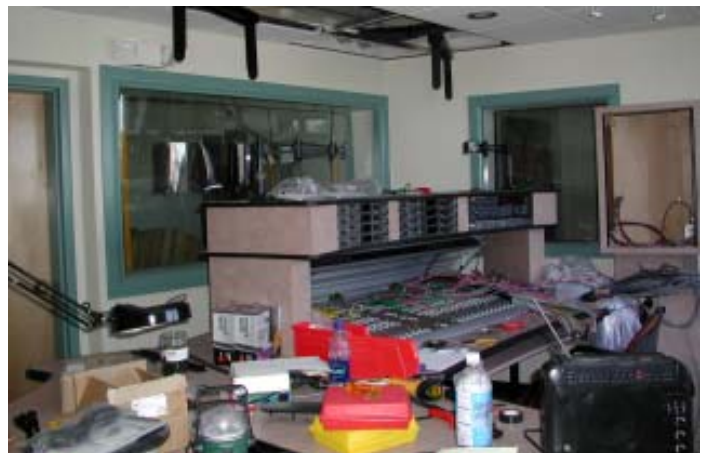
The new control room (some assembly required).
